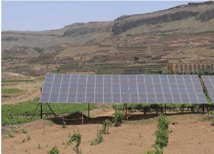
Figure 8: Solar power electricity for agricultural irrigation in Yemen.
